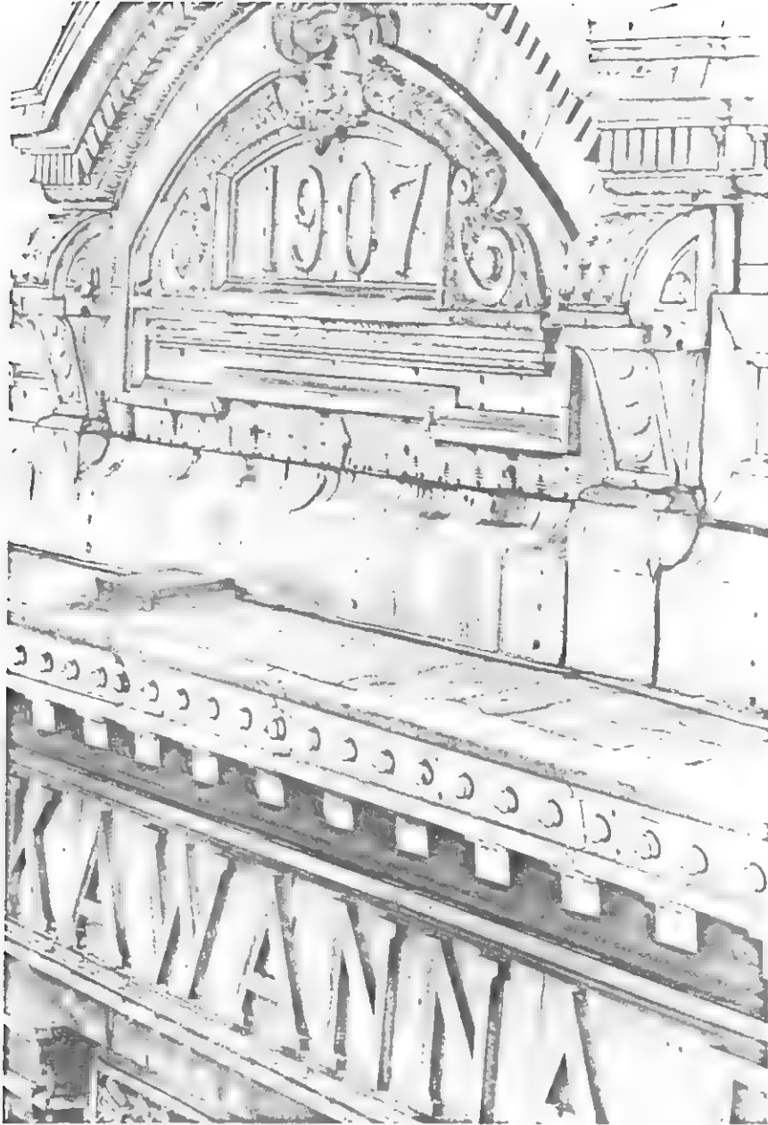
Detail in segmental arch over waiting room facade, giving completion date of terminal.
